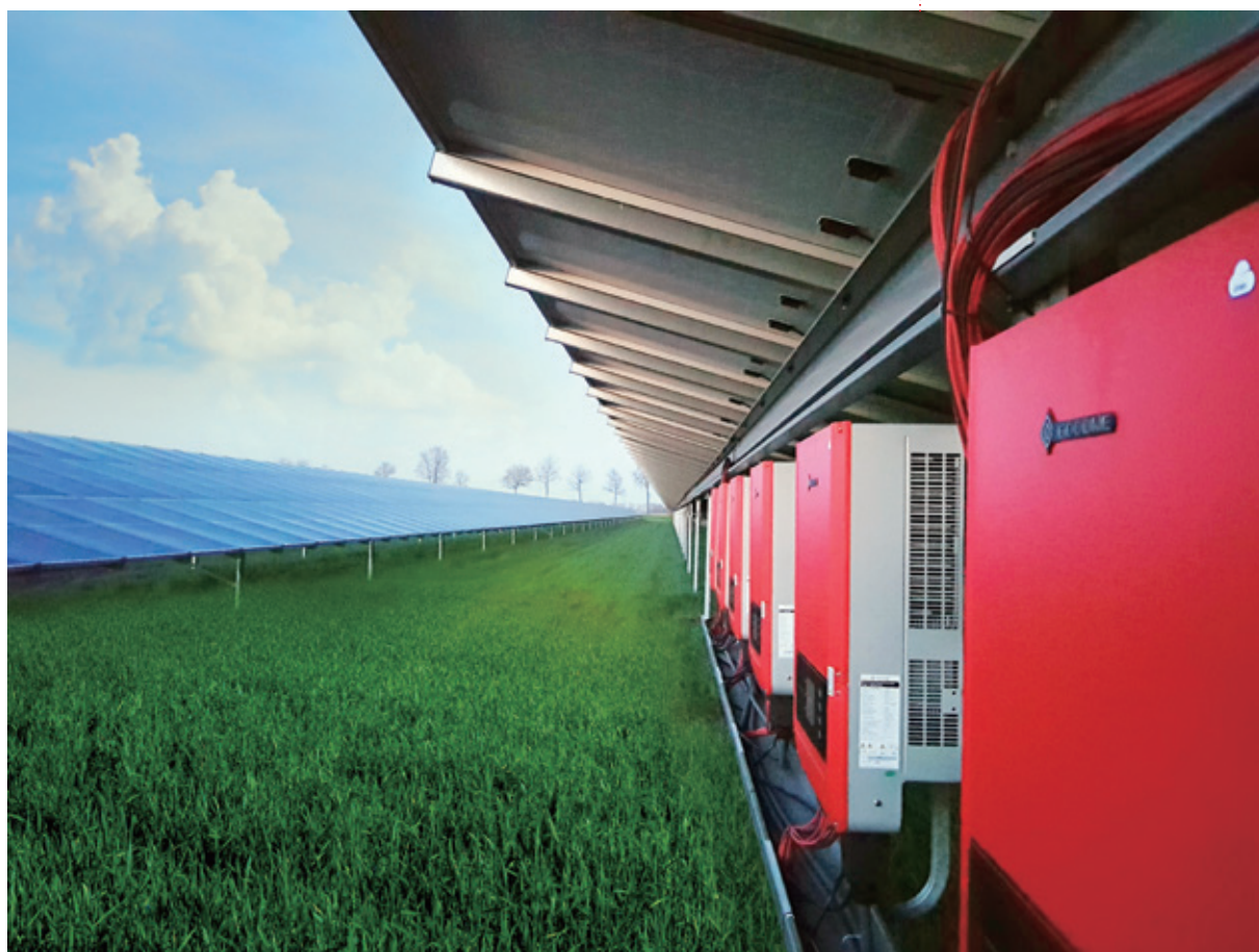
12MW Rotterdam | Holanda
