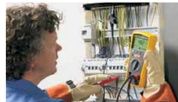
Insulation test at a distribution panel
